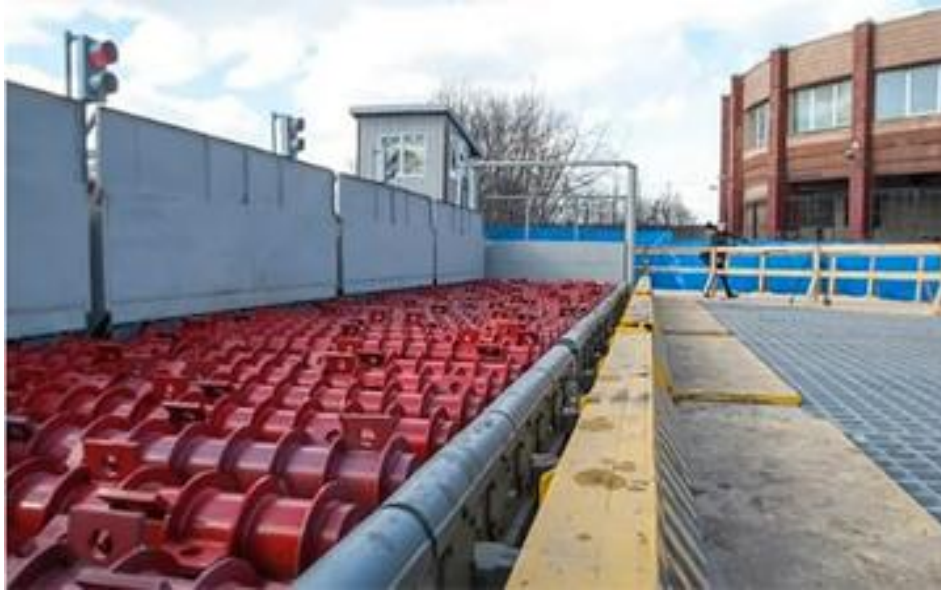
Figure 2. Snow melting complex with crushing plant
