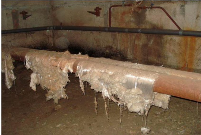
Figure 1. Disturbance of the thermal insulation of the pipeline
